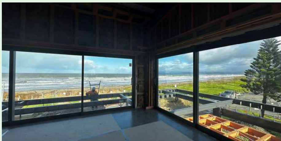
Up to 6m wide decks in places, spanning a total of 100m on three sides of the development making the most of the breathtaking views and the famous Gizzy sunset.
