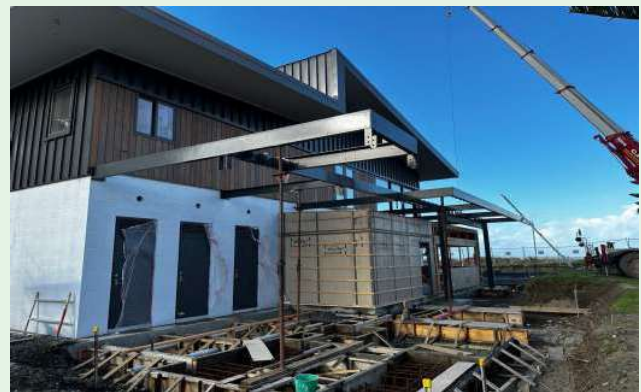
Up goes the steel work for the sweeping decks above the kiosk
