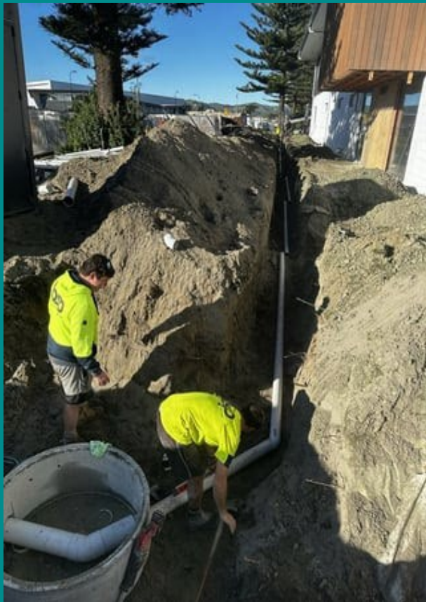
Good drainage and plumbing is key
